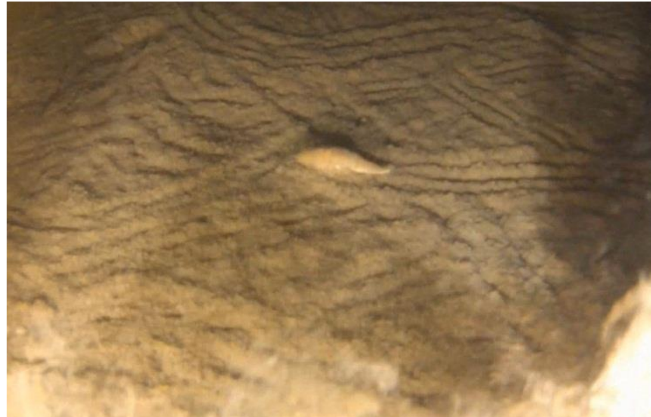
soft mud accumulated in the area of concretions extraction
